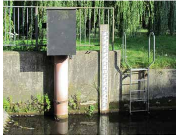
A water gauge on the River Cray at Hall Place Gardens © Rory Walsh
